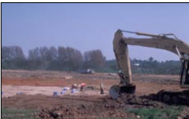
Excavation work taking place prior to the building of the Channel Tunnel Rail Link. Image Copyright Union Railways (South) Ltd.
